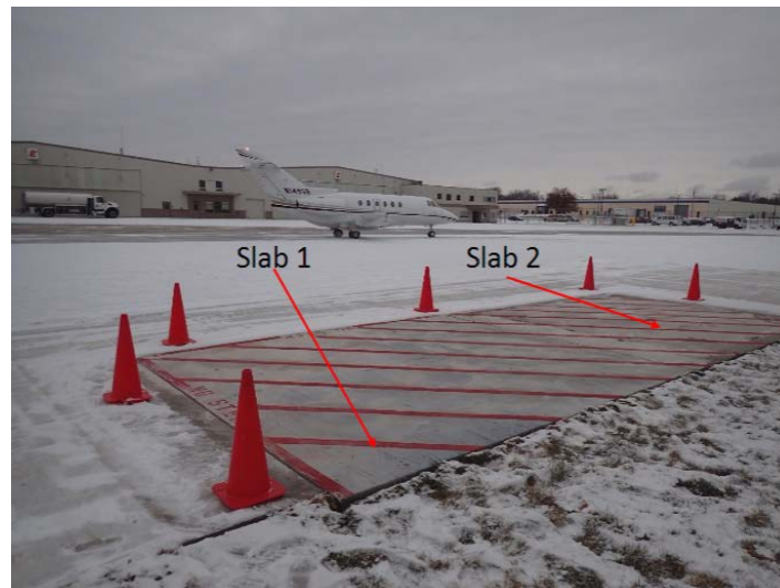
Figure 2-1 Electrically conductive concrete (ECON) test slabs built at Des Moines International Airport (DSM) (photo taken December 23, 2016)
