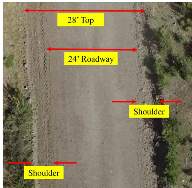
Figure 6-2 Gravel road cross section used in the analysis (photo taken on September 23, 2017, at Cherokee County, IA, U.S.A.)
